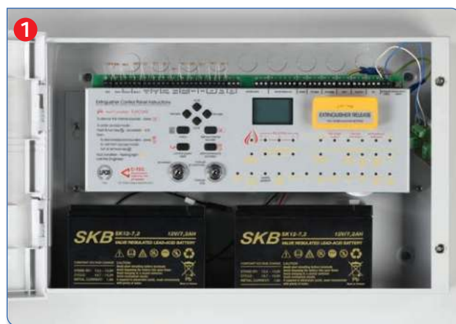
Automatic extinguishing unit
